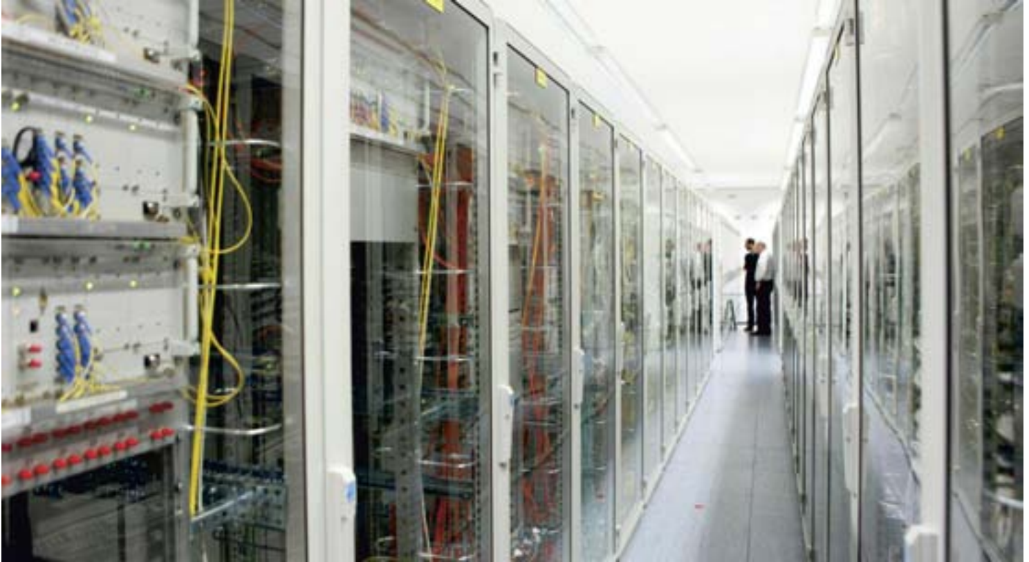
The Server Center – processing customer and product data for the new Commerzbank
